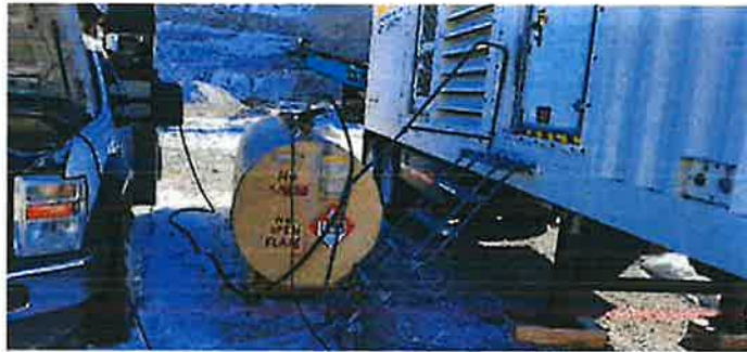
1000 - gallon fuel tank
