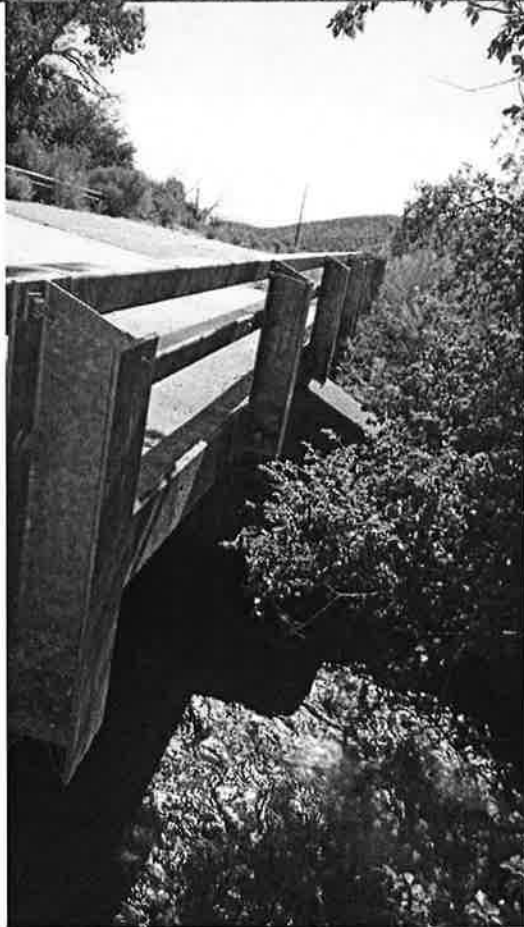
Site 1: Lower Location – Pine Creek Road (note lack of curb)
