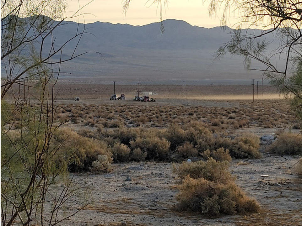
Photos of Dust Emissions from REP 2021-01 Construction on December 6, 2021 provided to Inyo County Planning Department and Great Basin Unified Air Pollution District
