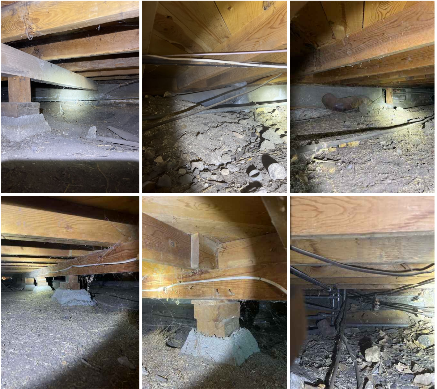
most of the wiring is running under the home
