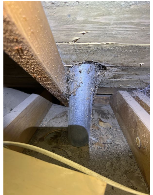
Water heater vent
