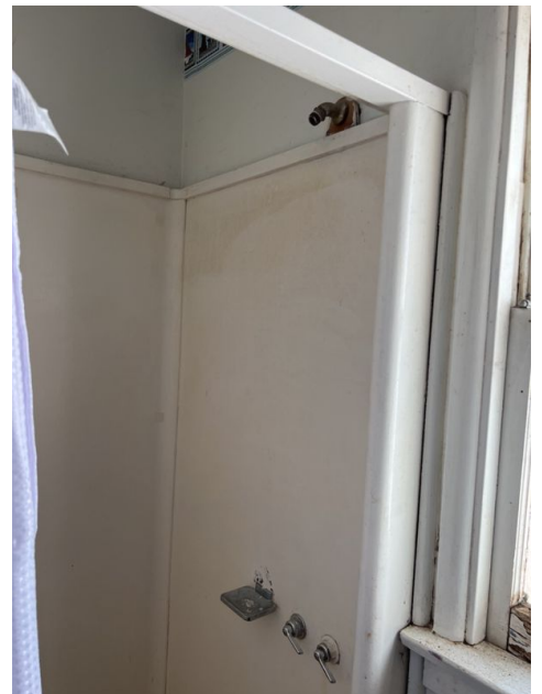
Water was off for the shower
