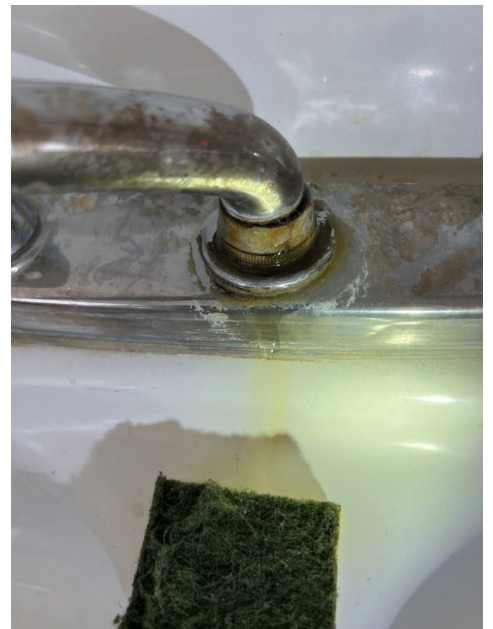
It was leaking under the sink
