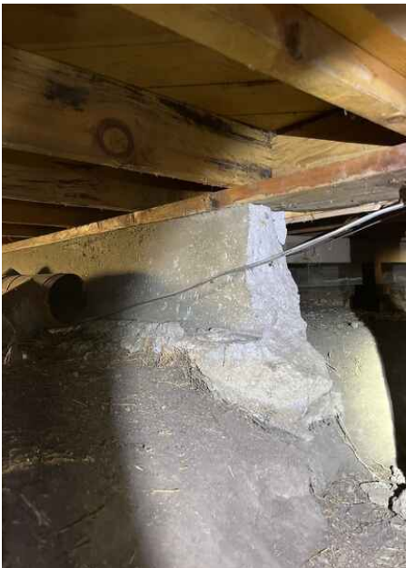
The foundation wall depth is typical of the era though not as deep as modern homes
