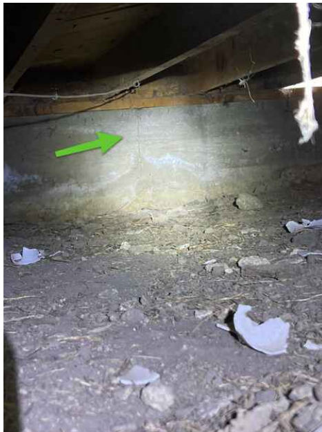
There was a crack observed at the SE corner of the foundation wall, viewed from the crawlspace there was no displacement and this crack is not a concern. Keep an eye on the crack at the exterior and consult a contractor if it grows rapidly
