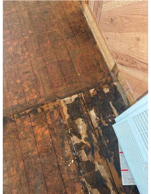
mastic on floor, living room
