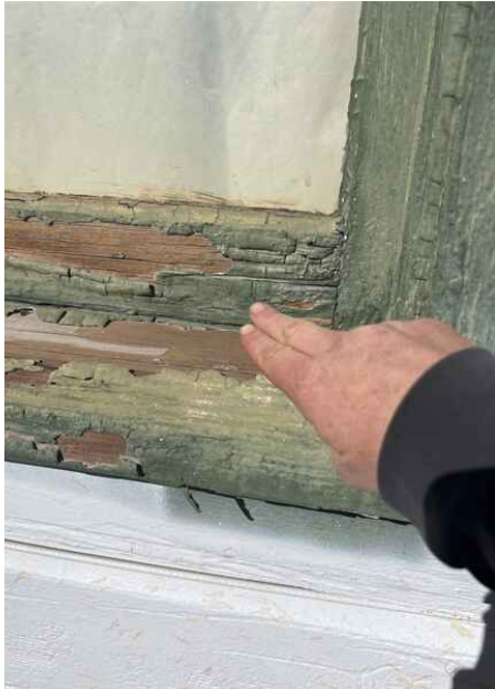
paint at window trim, south side
