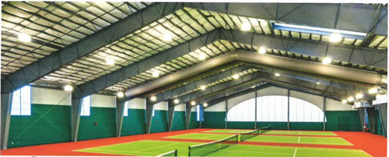
Pre engineered metal building interior showing compressed insulation.
