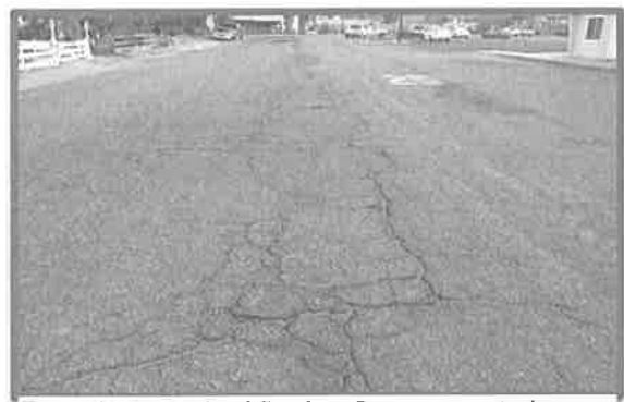
Figure 3 Example of Cracking Pavement, typical
