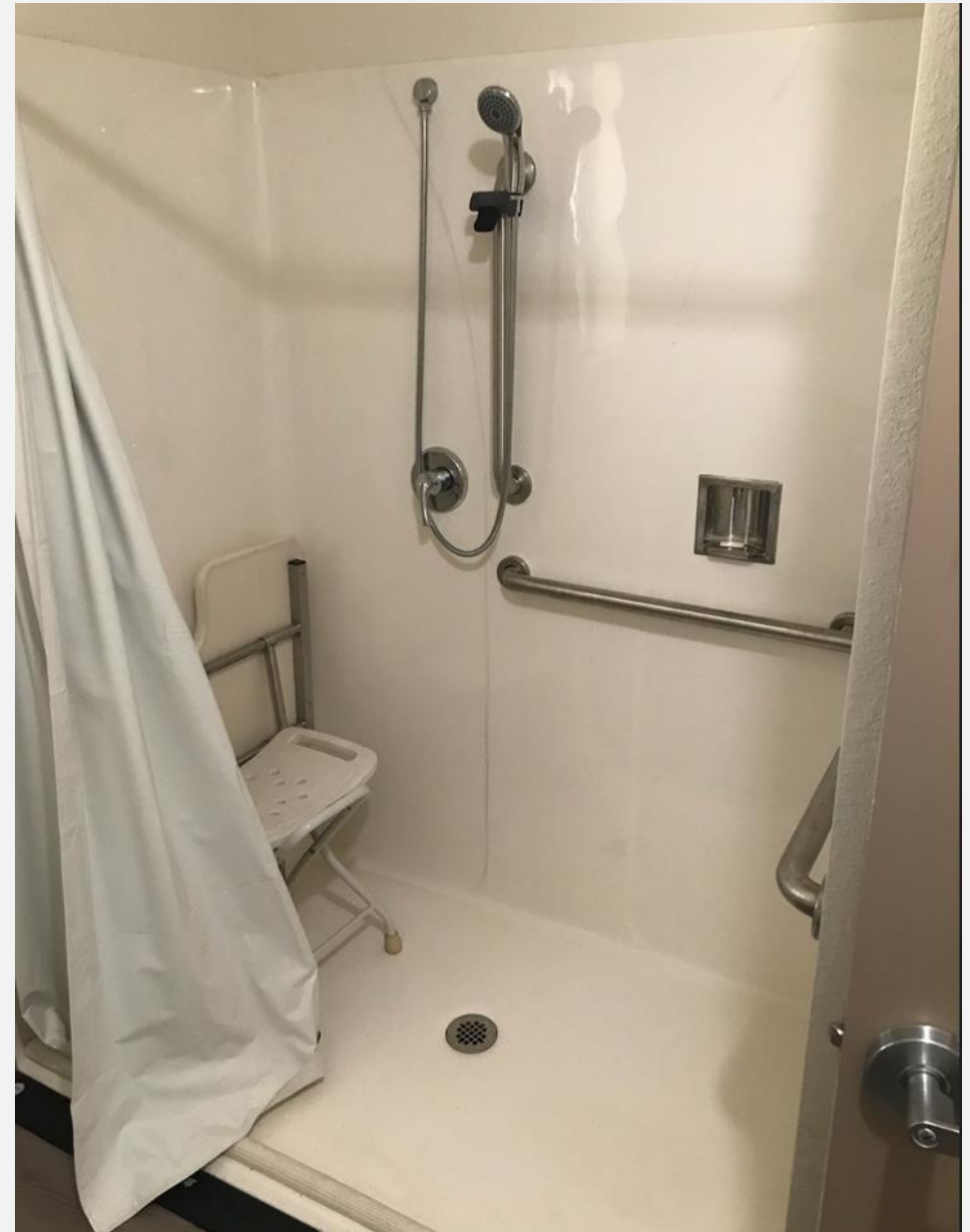
The bathroom at Bishop Senior Center was remodeled to comply with ADA Standards.
