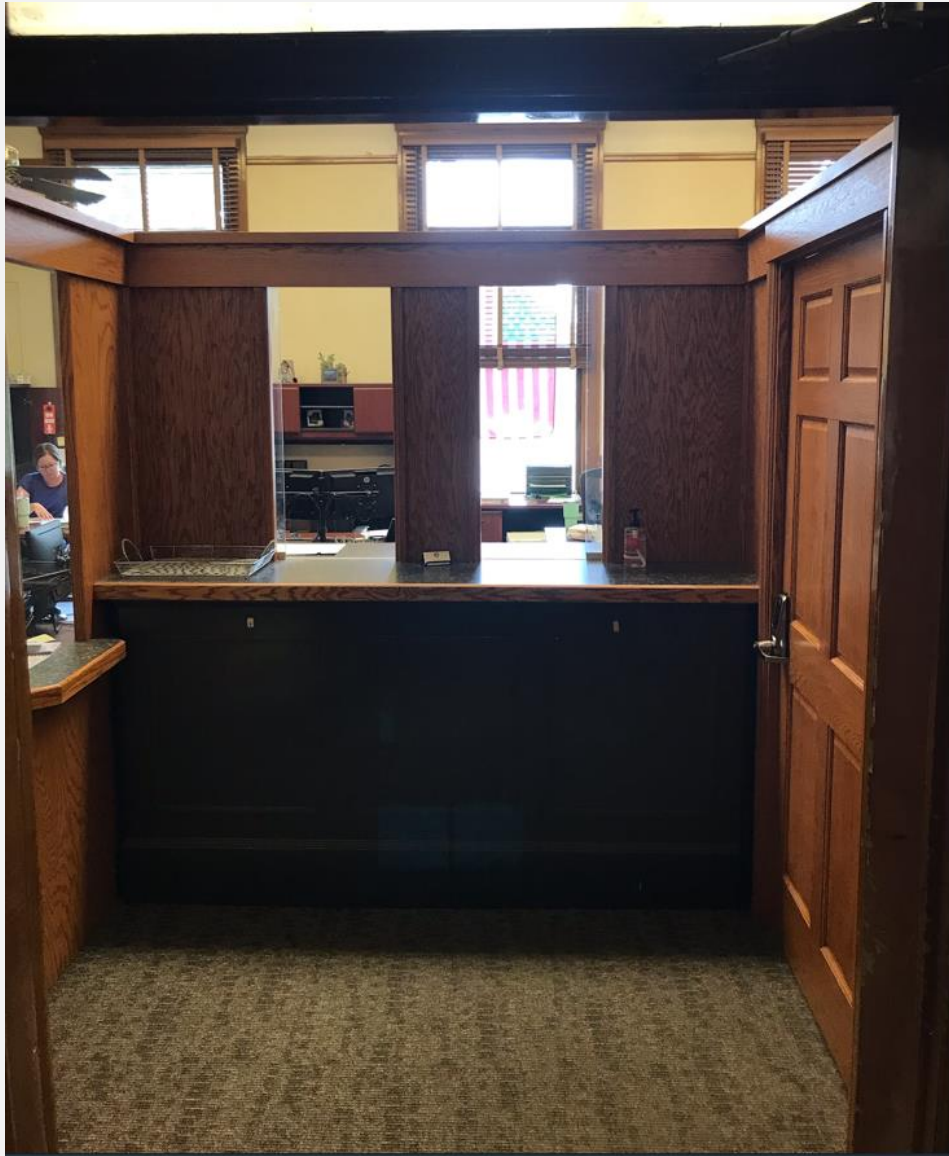
The B&M Team built and installed the new security panels in the office of the auditor.
