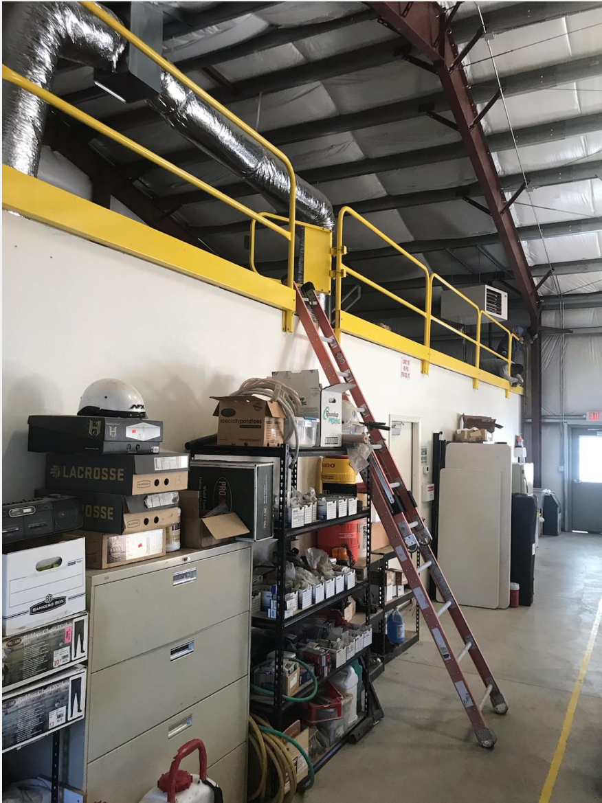
New Safety Guardrails for the Ag building mezzanine were installed by B&M.
