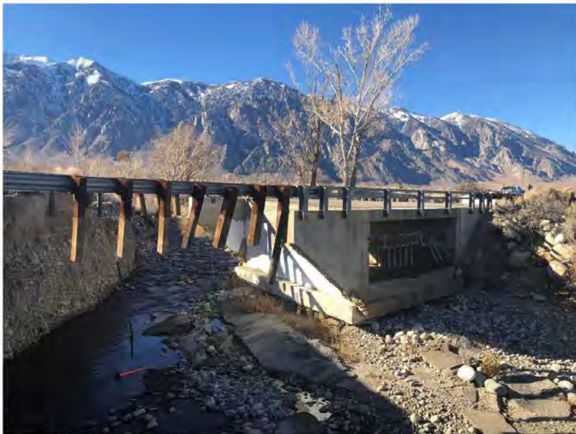
View of existing failed bridge over Pine Creek and abutment to be removed.
