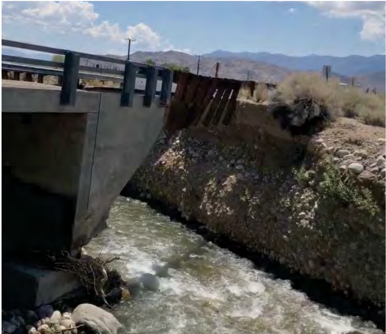
Figure 5 – Failed South Abutment, 2018
