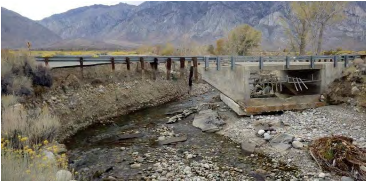
Figure 1 – North Round Valley Road with failed south abutment (looking west/upstream)
