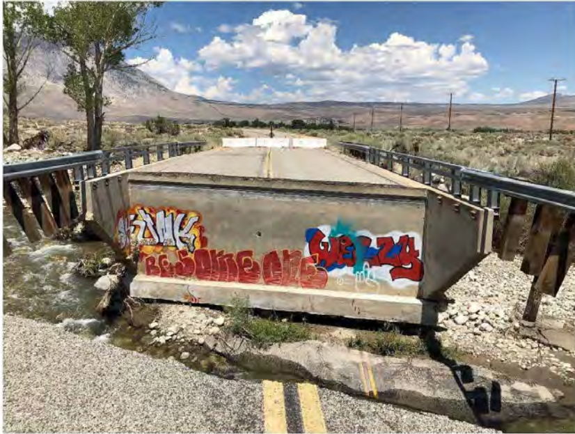
View of existing failed bridge over Pine Creek. A portion of the existing bridge abutment is located within the OHWM of Pine Creek.
