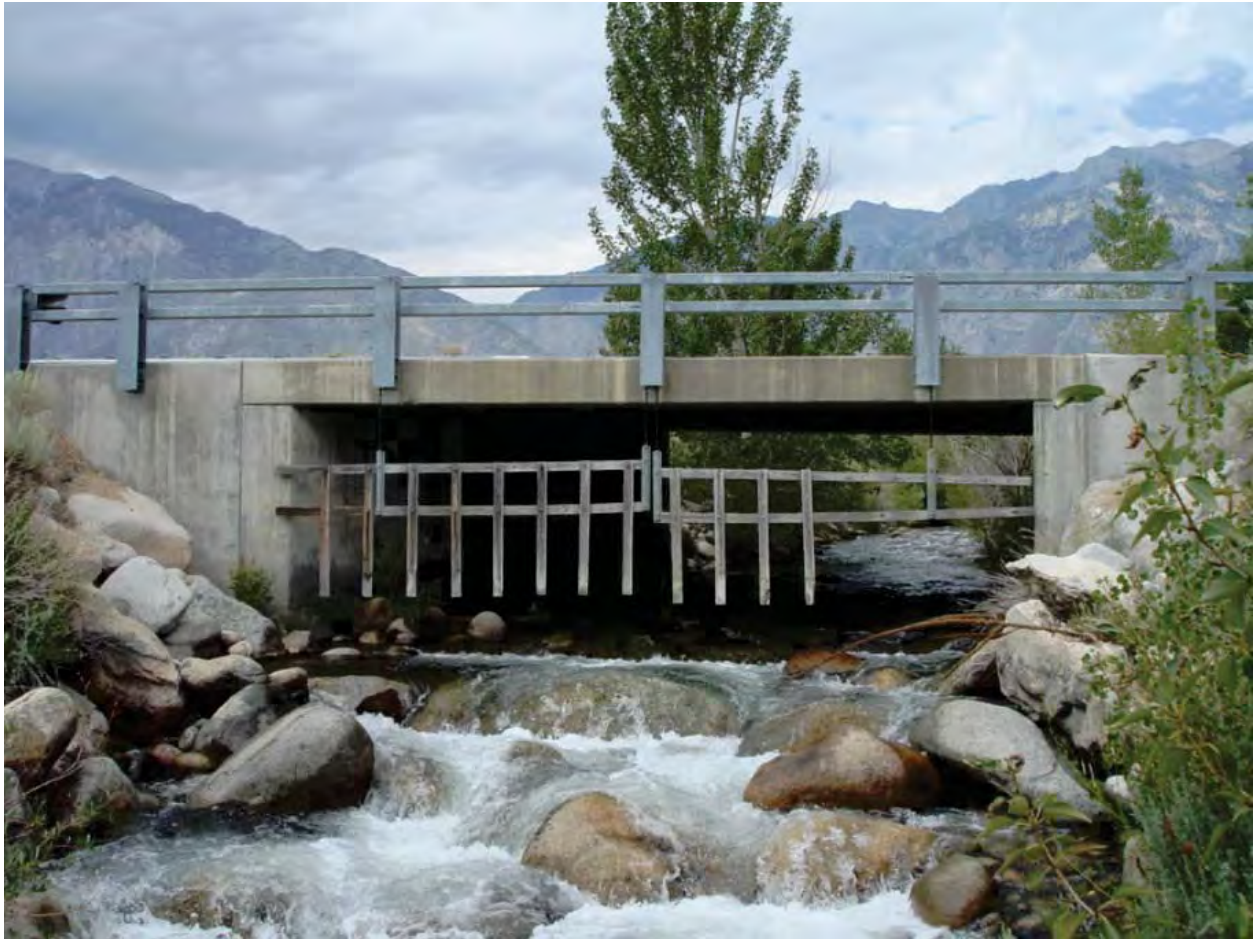
Figure 4 – Downstream Face with Grade Control prior to Failure, 2008
